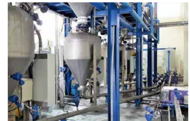
输送系统现场图 Conveying System
