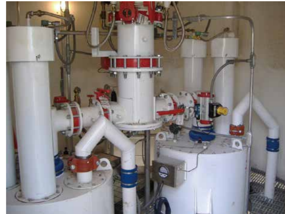
➤ 失重式计量站 Loss-in-weight Dosing Station
