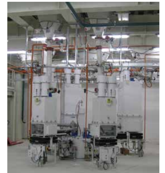
Loss-in-weight Dosing System ➤ 失重式计量系统现场图
