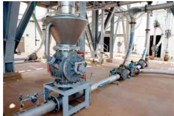
➤ 现场图 Installation Site
